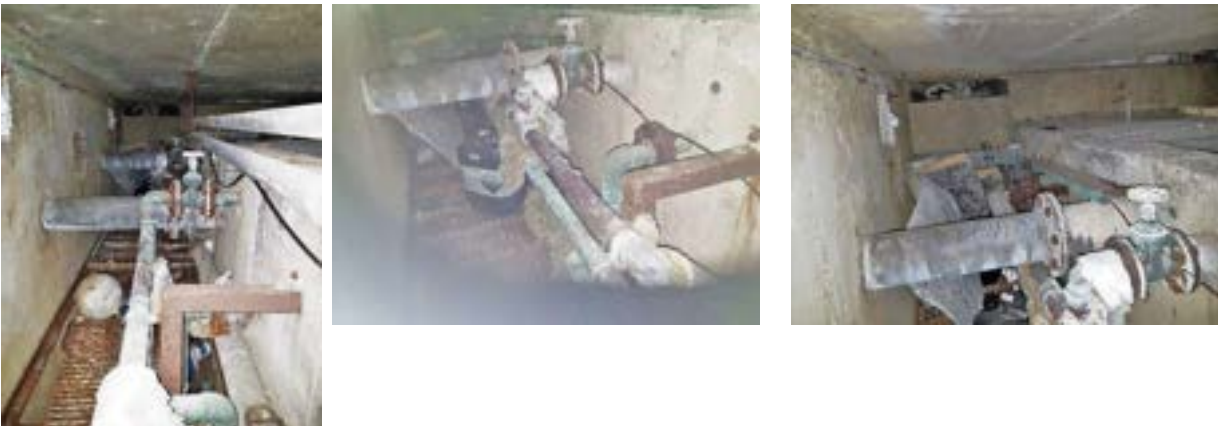
The two mains cold water supplies where they connect to the ball valves in the tanks. The rotten walkway, the abandoned and rubbish materials including chemicals. The level of dust and dirt presents a serious health hazard and the area must be considered a confined space.
