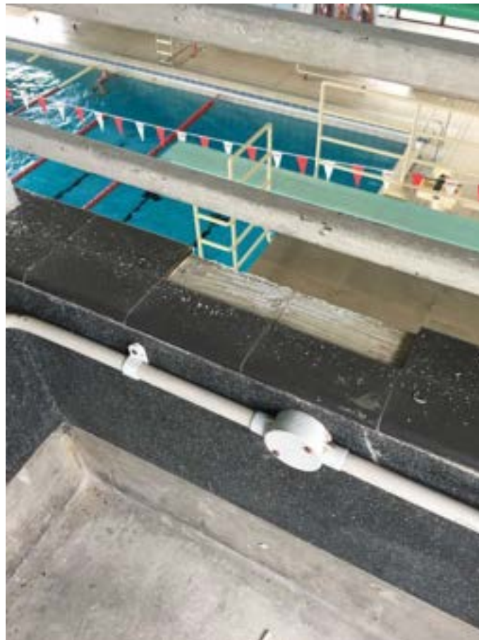
Fig 4.4.7 – The photo above was taken within the main pool area on the second-floor galleries showing a close-up view on the existing broken / missing tiles on the gallery parapets.
