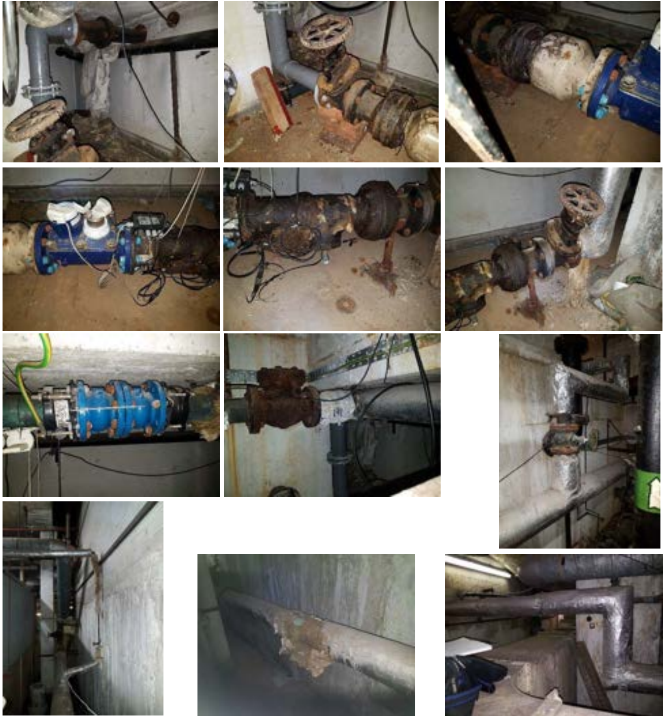
The incoming mains cold water service in cast iron, ABS, cast iron and mild steel. Note the inlet and outlet valves supported on bricks and timber. The mass of Denso tape appears to be to mask a leak. The inaccessible double check valve, an old non-return valve that should have been removed and an original isolating valve. The mains cold water service pipework on the eastern wall of the plantroom and rising to serve the plantroom sink.
