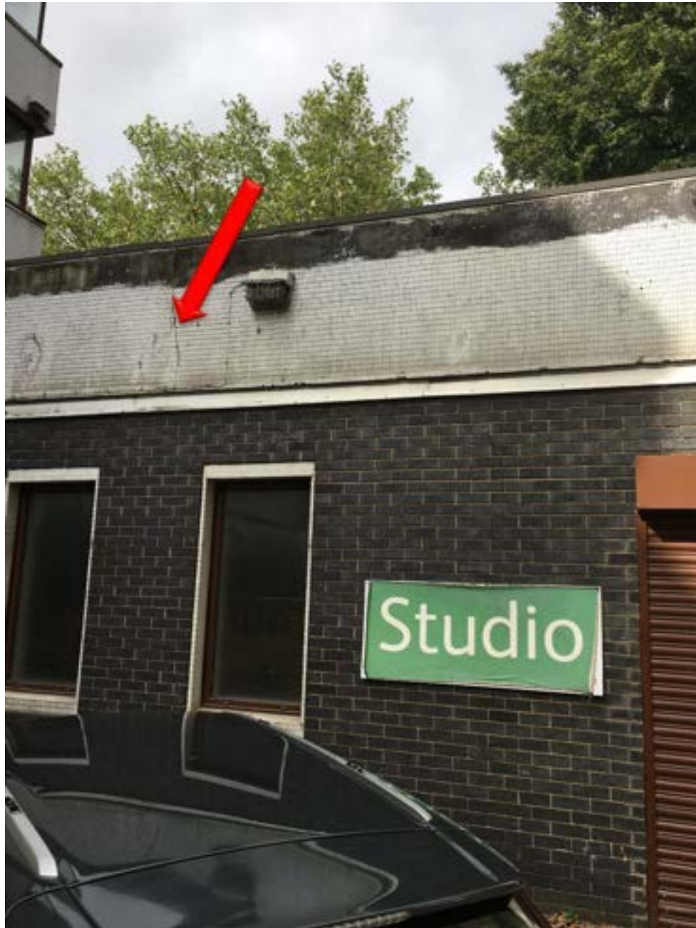
Fig 5.3 – The photo above shows cracking and movement to the rear roof parapet edge together with possible risk of mosaic tiles being shed.
