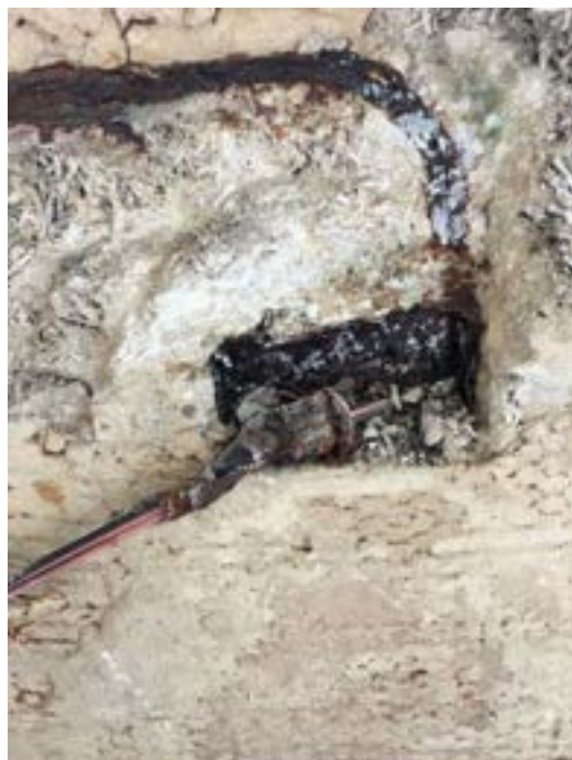
Fig 4.4.5 – The photo above was taken within the main pool area on the second-floor galleries.
