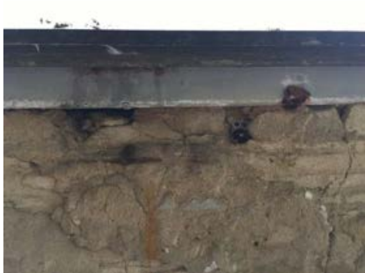
Fig 4.4.6 – The photo above was taken within the main pool area on the second-floor galleries showing a close-up view on the existing wall to window interface.
