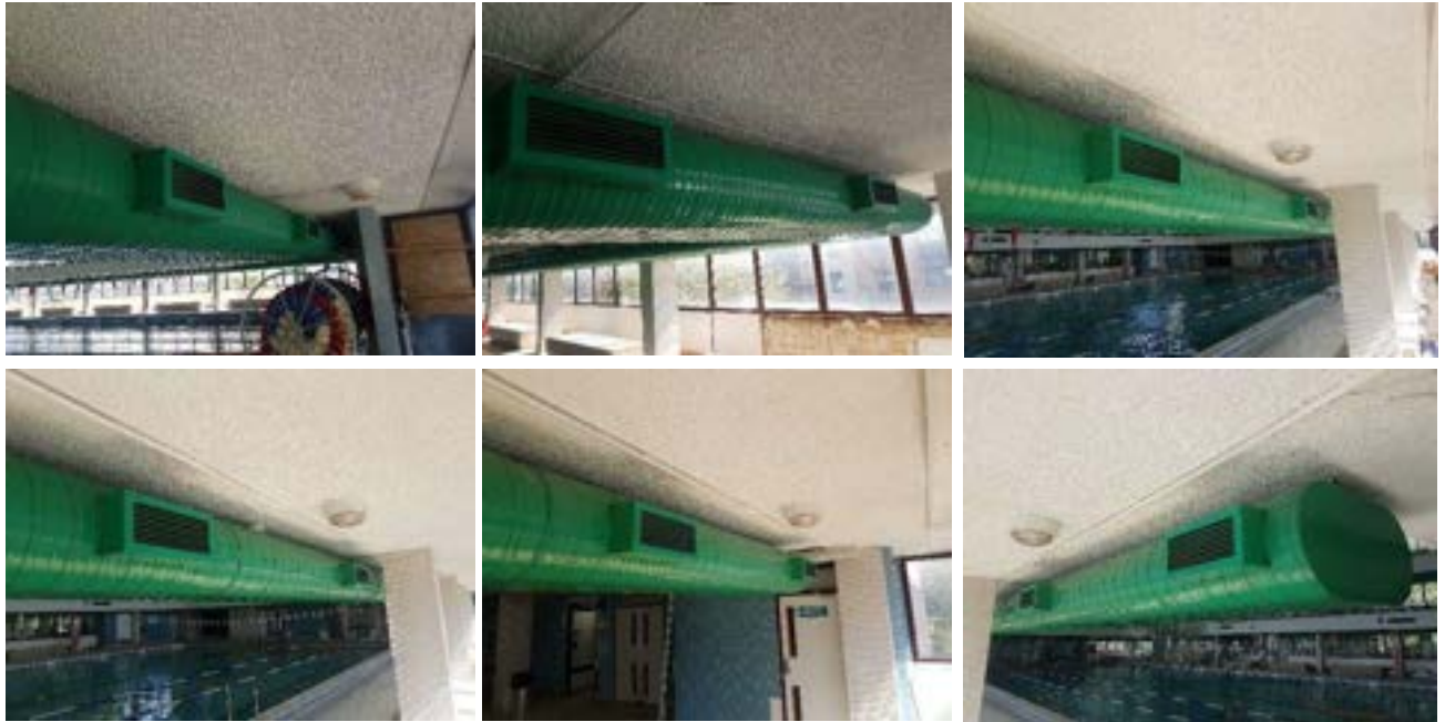
The supply air ductwork around the 1 st floor level of the main pool hall. The dirty grilles are most probably a reflection of the interior of the ductwork as well and all need cleaning.
