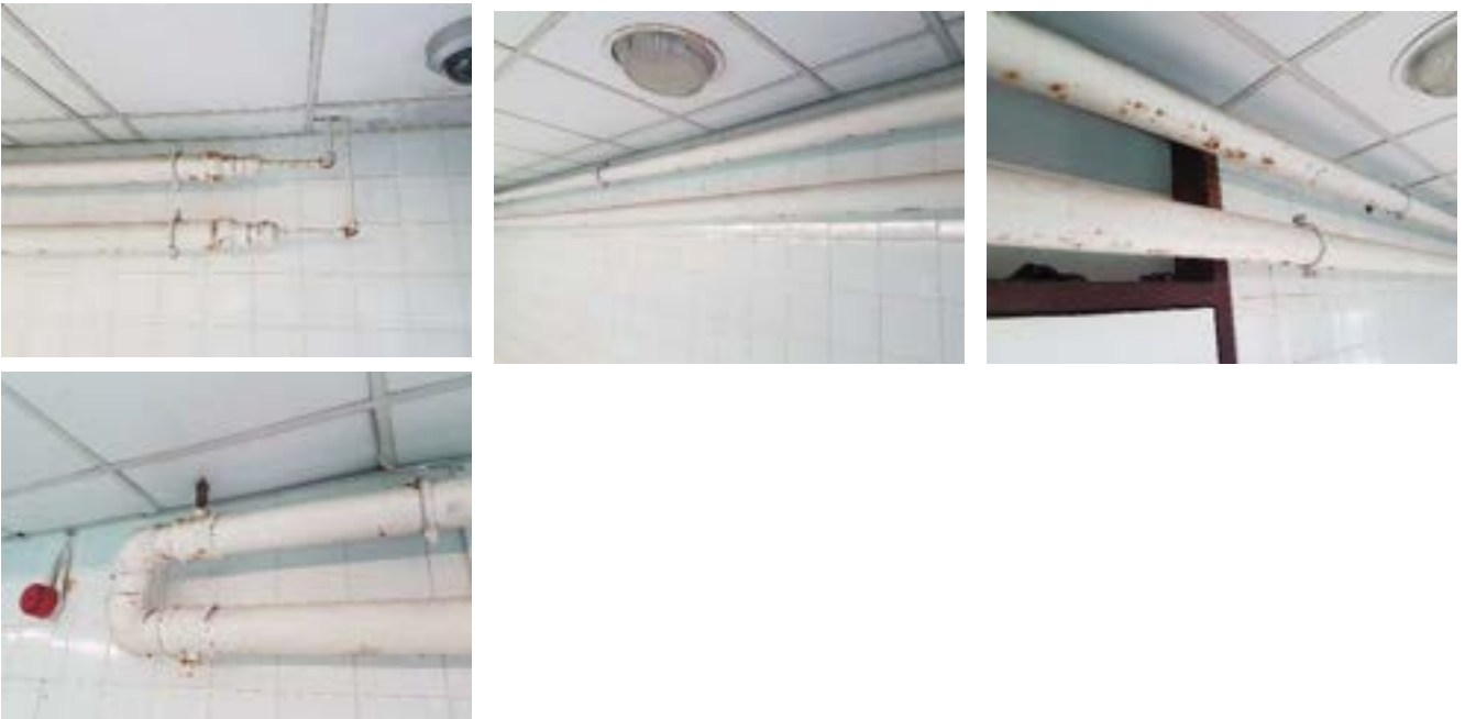
The tubular heating coil at the east end of the teaching pool and the leg that sits at high level on the north wall. The corrosion of this heating coil is starting to appear.
