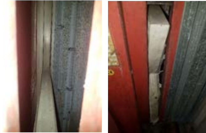
The upper filter chamber with no filter installed. The lower filter chamber showing the heavily soiled and damaged filter which was unremovable.
