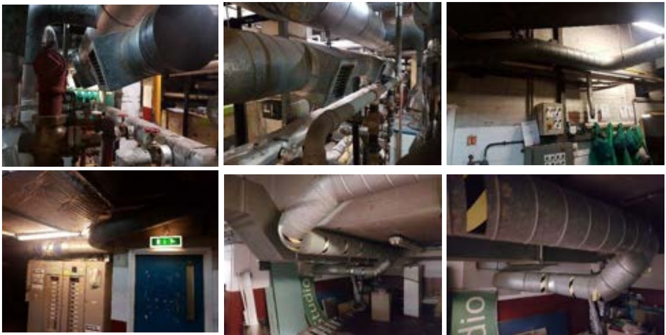
The boiler combustion air extract system showing the 3 no. grilles above the boilers, the ductwork at high level, the cased axial extract fan located above the main electrical distribution for the building and where the system enters the old fresh air plenum.
