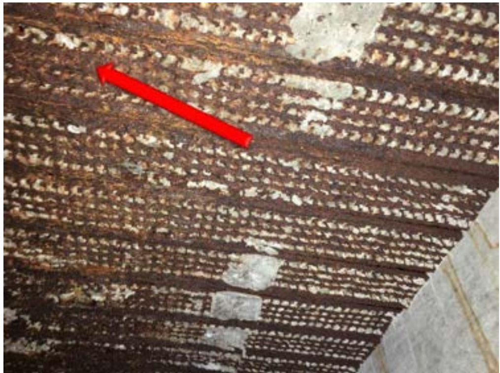
Fig 4.4.1 – The photo above was taken within the main pool area on the second-floor galleries.
