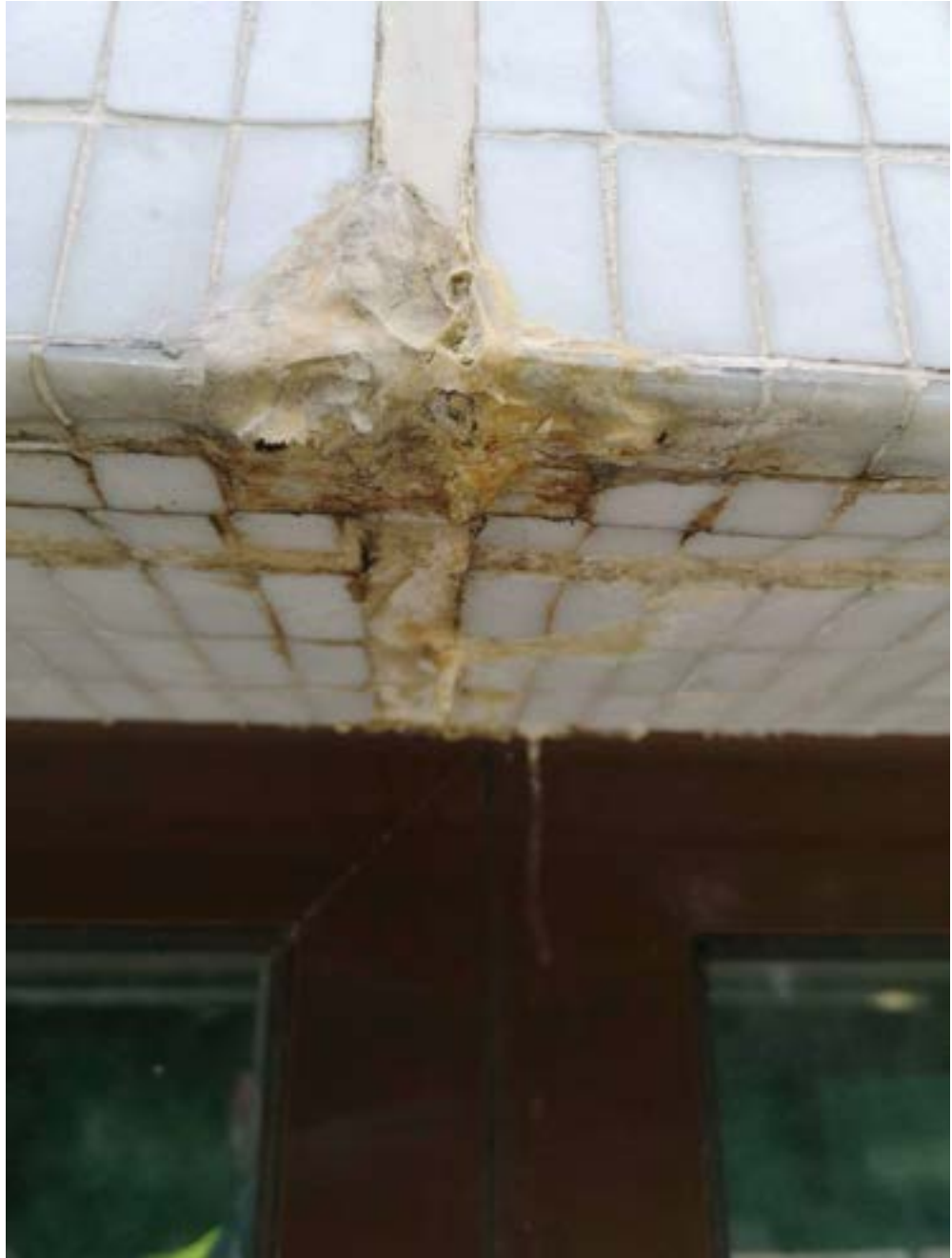
Fig 5.2 – The photo above shows a typical example of potential tile shelling at movement joint in the façade and an historic repair.
