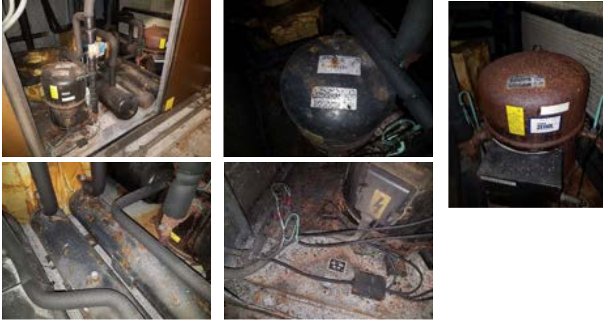
The non-operational refrigeration/de-humidification section. There is a high level of corrosion to both the casing and the equipment & wiring.
