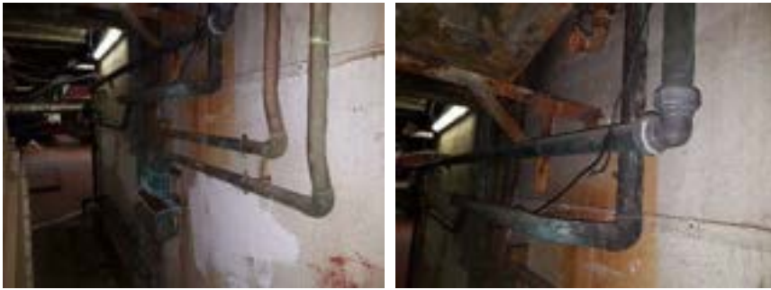
The two mains cold water supplies, one raw water and one softened water, pass along the wall before rising to the tank room.
