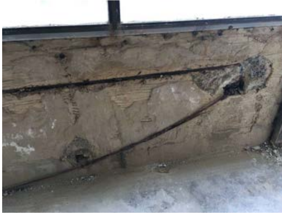
Fig 4.4.4 – The photo above was taken within the main pool area on the second-floor galleries.
