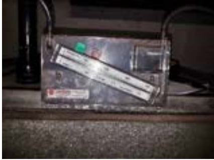
The filters have a pressure loss manometer fitted across them but this without any fluid
