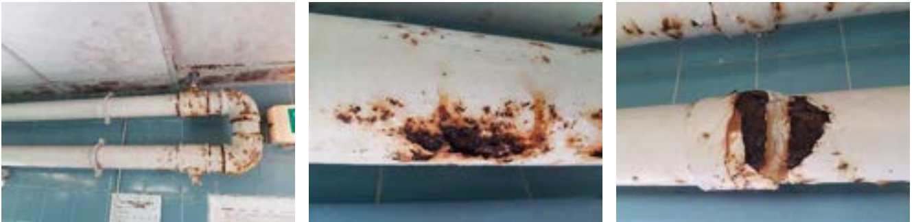
The tubular heating coil at the east end of the teaching pool and the leg that sits at high level on the east wall. The corrosion of this heating coil is very bad.
