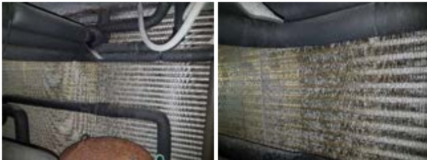
The de-humidification coil is very heavily corroded and the internal condensate drain channel was blocked.
