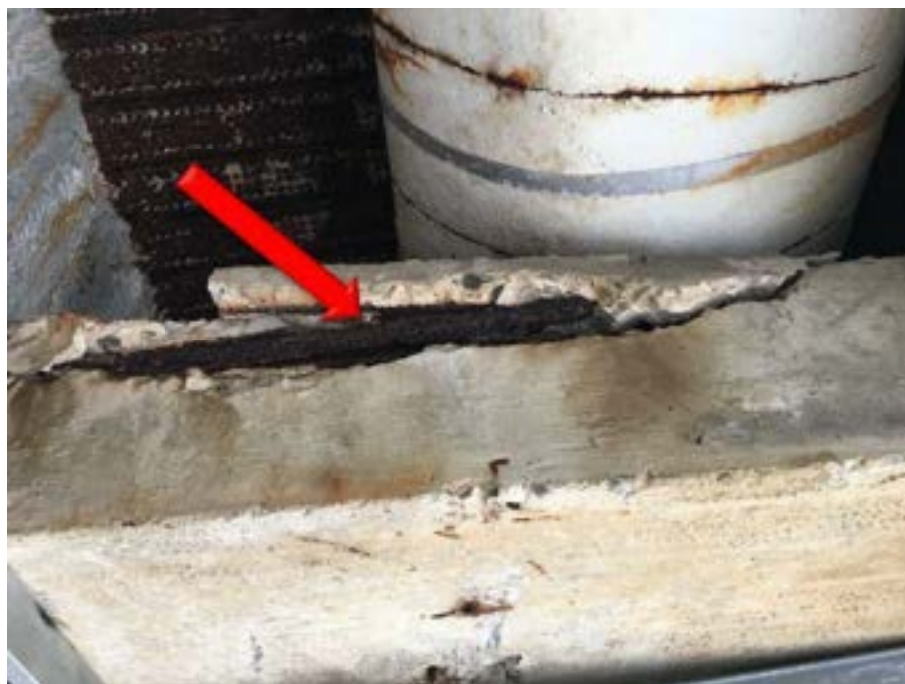
Fig 4.4.3 – The photo above was taken within the main pool area on the second-floor galleries.
