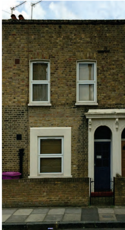
Loss of original cornice, windows, window mouldings and railings
