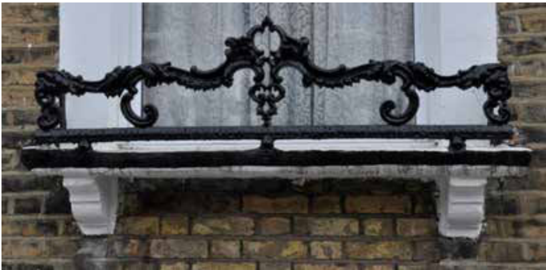
Different types of wrought ironwork window guards. Both of the above examples are from Driffield Road but these guards are also present on some properties in Ellesmere and Vivian Road.
