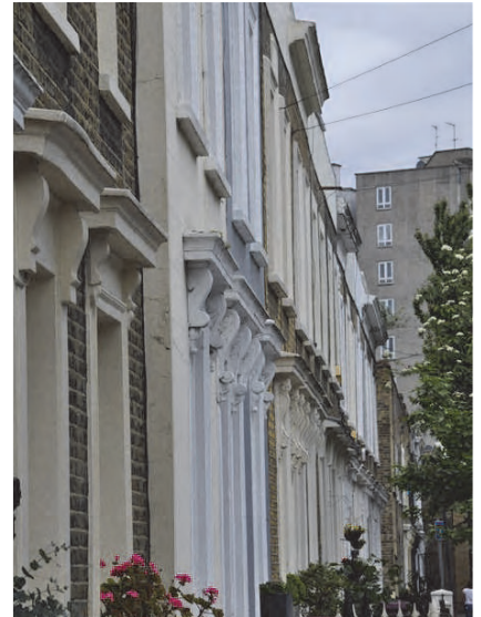
Loss of cornices reduces the rich character of the streetscape
