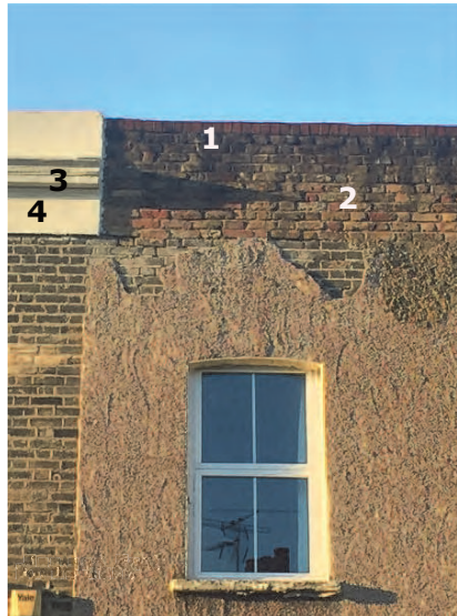
Cement coatings and lack of mortar can reduce the life of the brickwork
