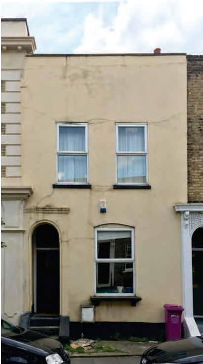
Removal of features and rendering the facade can result in significant loss of character
