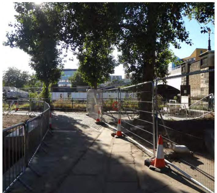
Right: Public realm being delivered on the east bank of Twelvetrees Crescent Bridge, due for completion November 2016
