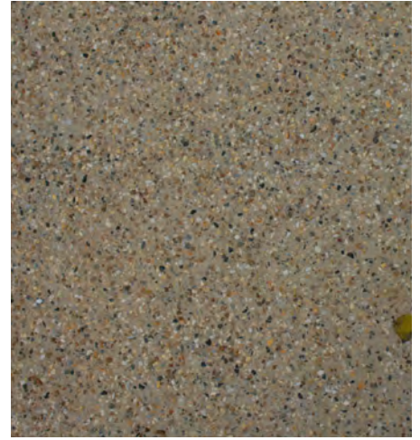
Spray tar and chippings repairs to existing asphalt pathway at Three Mills Green
