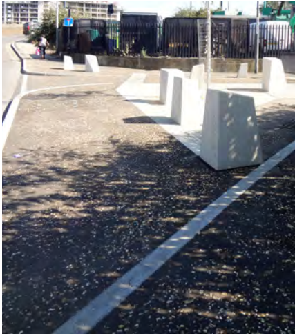
Example of standard asphalt distinguished by the use of river gravel aggregate
