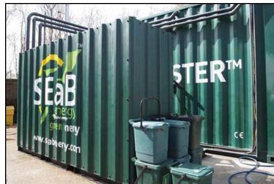
Image 10: Flexibuster & CHP unit
