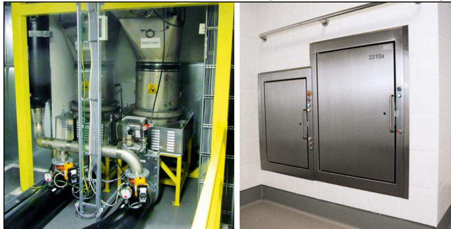
Image 6: Inlet doors and basement mechanism for systems installed into buildings
