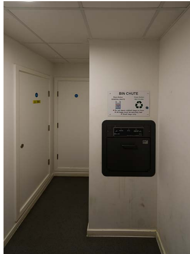
An ineffective waste chute. It is not located in a special room, signage is unclear, the area lacks ventilation and the surrounding area would be easily damaged if waste was left on the floor.
