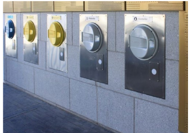
Fig. 14. An example of an AWCS portal area, demonstrating ease of access. Image courtesy of Envac.
