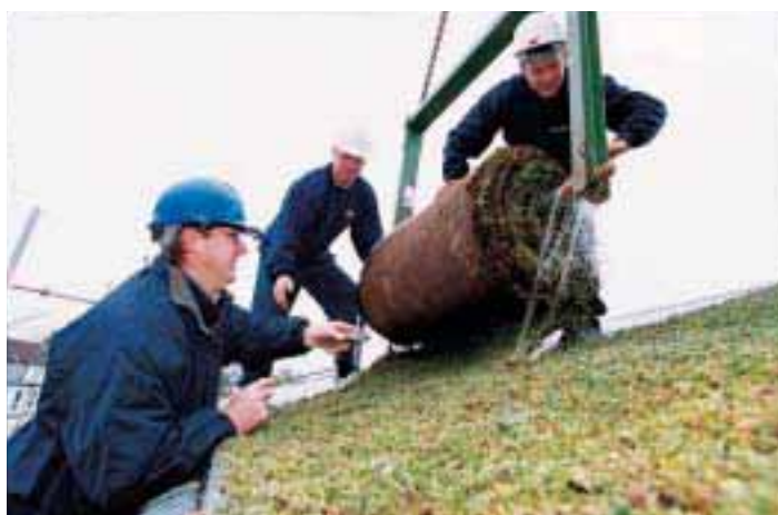
Laying the Sedum Roof on eco semi detached home in East London. East Thames HG
