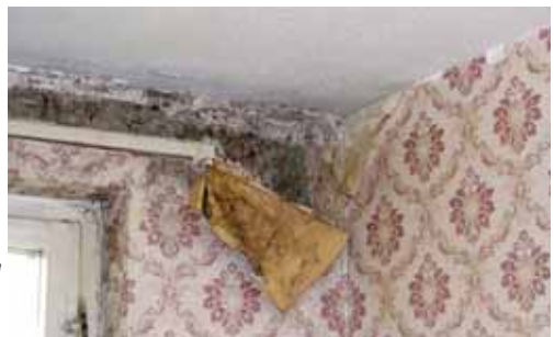
Damage to decorations caused by condensation.
