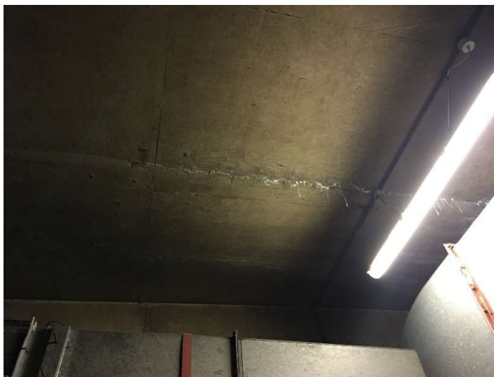
Examples of water seepage through original construction joints
