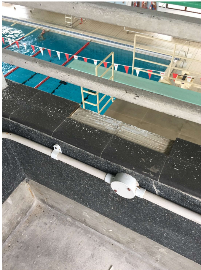
Close up missing / broken tiles on the parapets See CCLLP Drawing 18003-301-R for locations.
