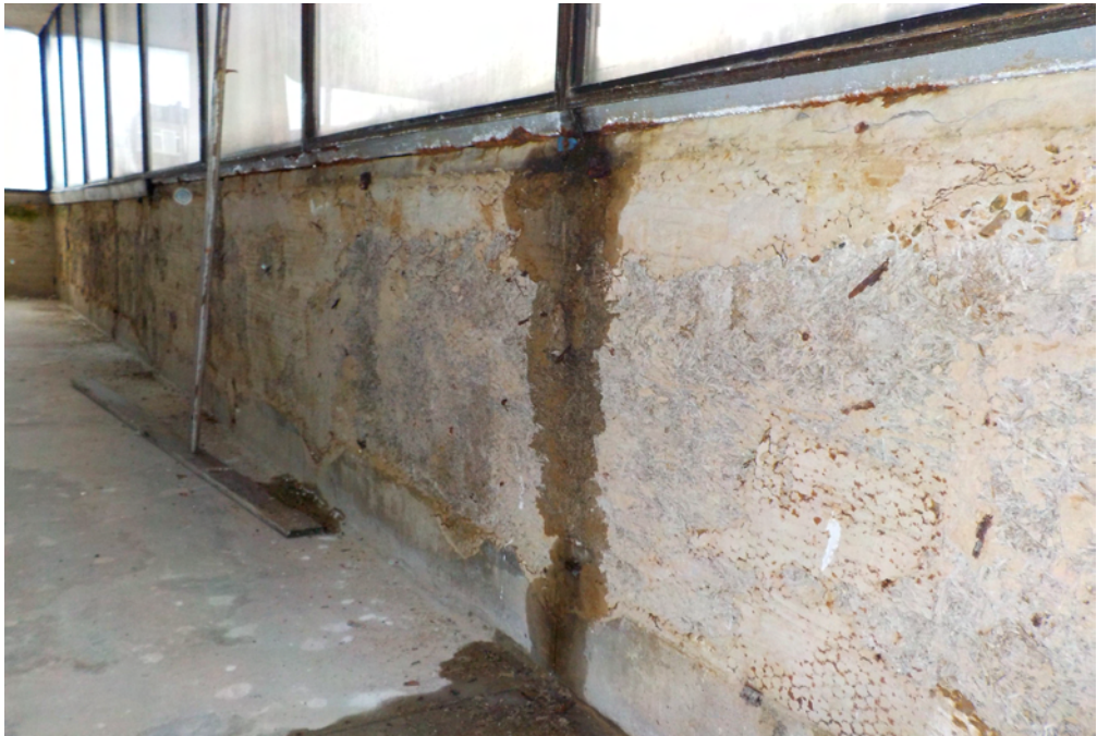
View of water penetration at spandrel wall / window interface It is likely that the window fixings have been affected by the water penetration with rust patches visible along the cill trim.
