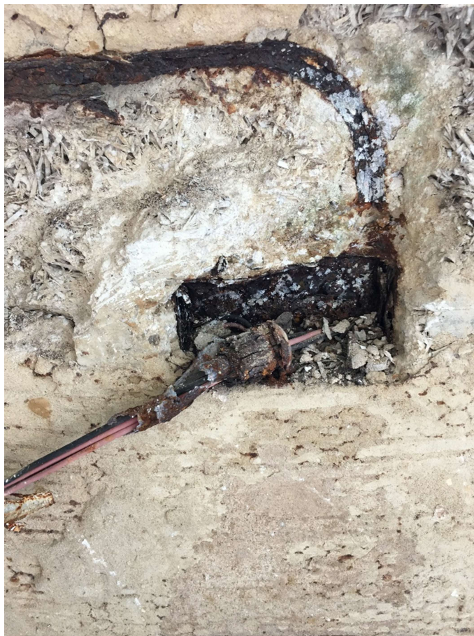
Typical views of Main Pool Hall spandrel wall 2 nd floor level Note: rusted electrical conduits and metal fixings in wall.
