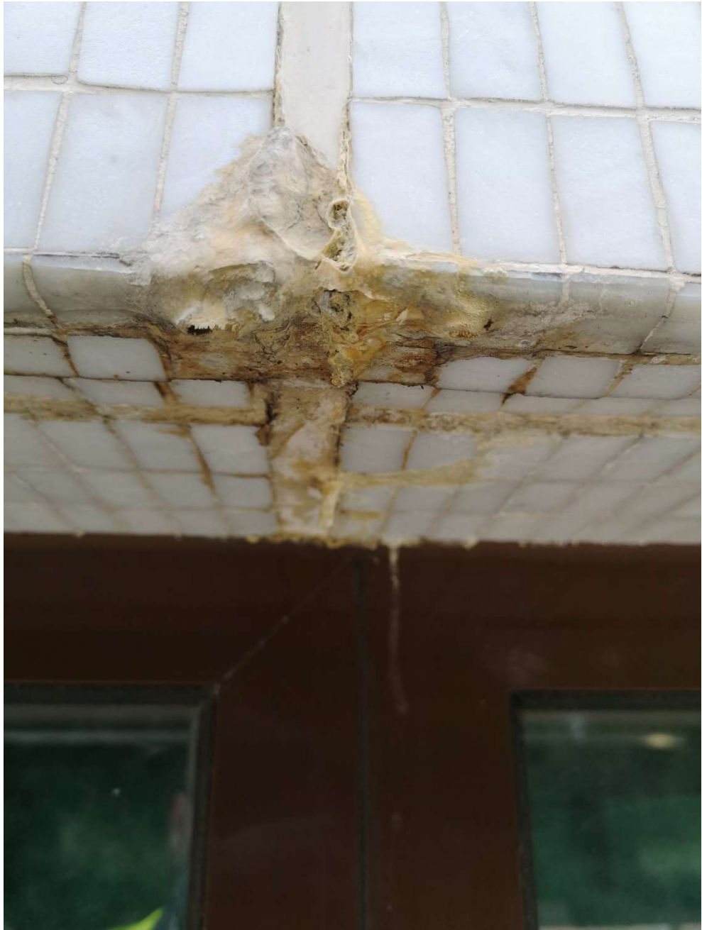
Movement joint in facade. The joint above shows signs of a previous repair.
