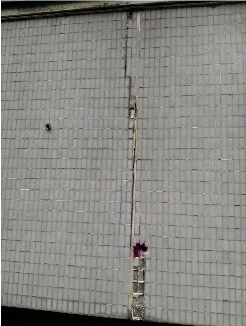
Typical example of potential tile shelling at movement joint in facade.
