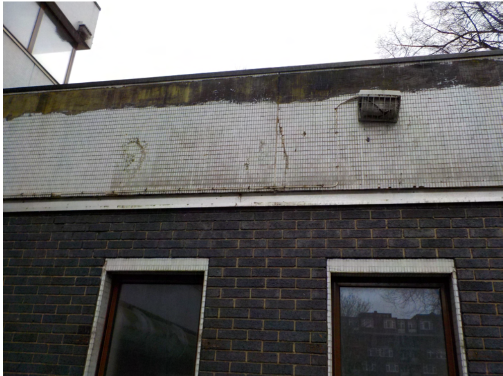
Example of cracking and movement to rear roof parapet edge together with possible risk of mosaic tiles being shed
