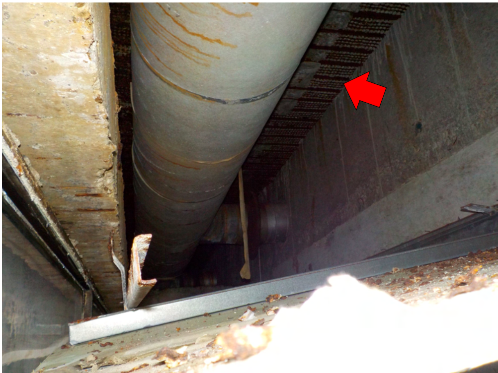
View above partially collapsing ceiling over 2 nd floor gallery It can be seen that the ceiling fixings on the left side have failed. Also note “Hyrib” roof slab reinforcement (arrowed).
