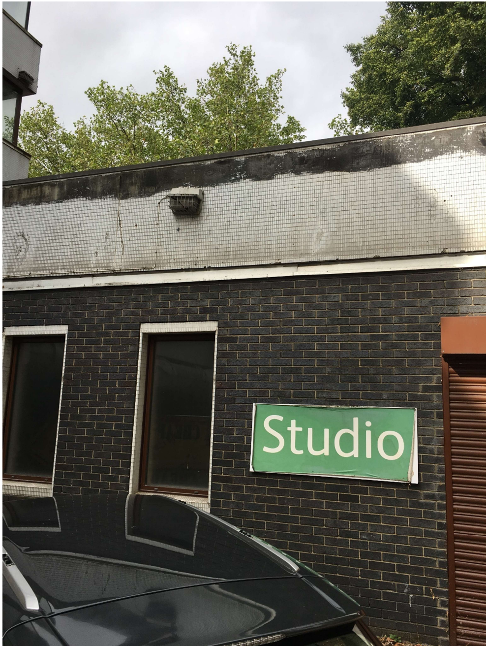
Example of cracking and movement to rear roof parapet edge together with possible risk of mosaic tiles being shed
